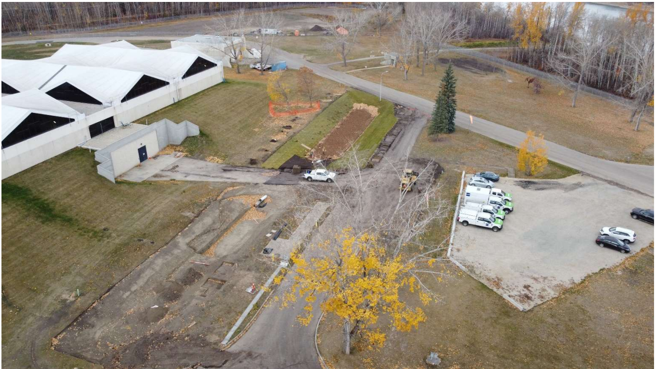
Figure 3: Low Impact Development at E.L. Smith, showing bioswales to collect and store storm water.
