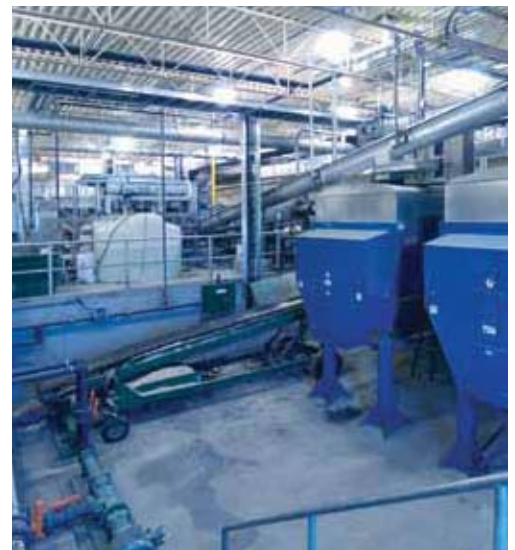
WWTP solids handling process equipment
