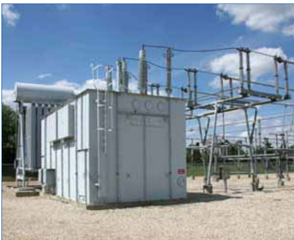
Example of a substation in an Edmonton community – with a transformer and connection equipment.
