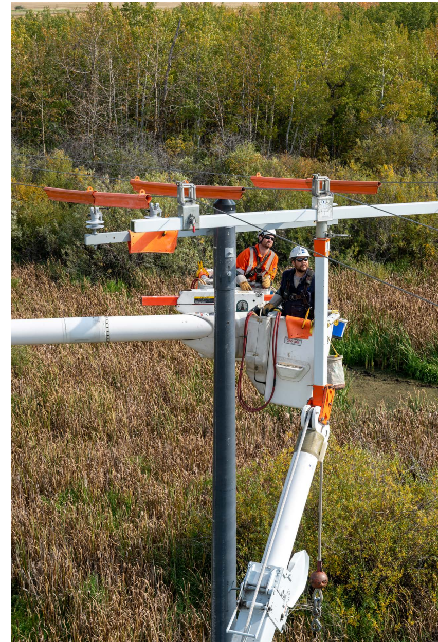
Electricity Services, Edmonton, Alberta, Canada
