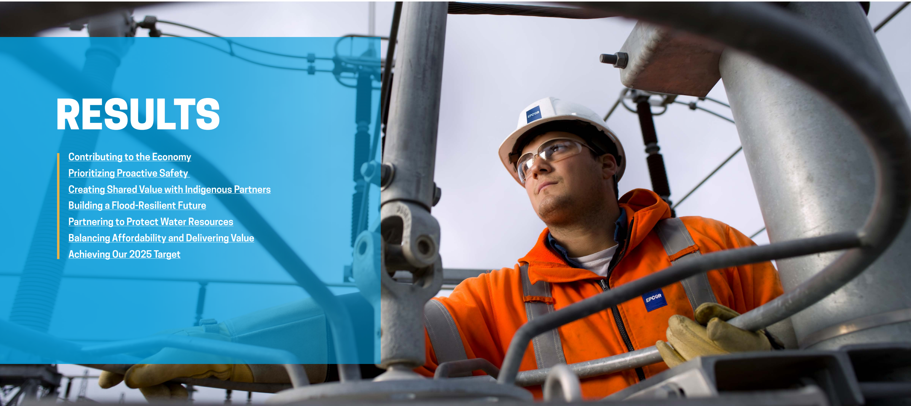
Electricity Services, Genesee Substation, Edmonton, Alberta, Canada
