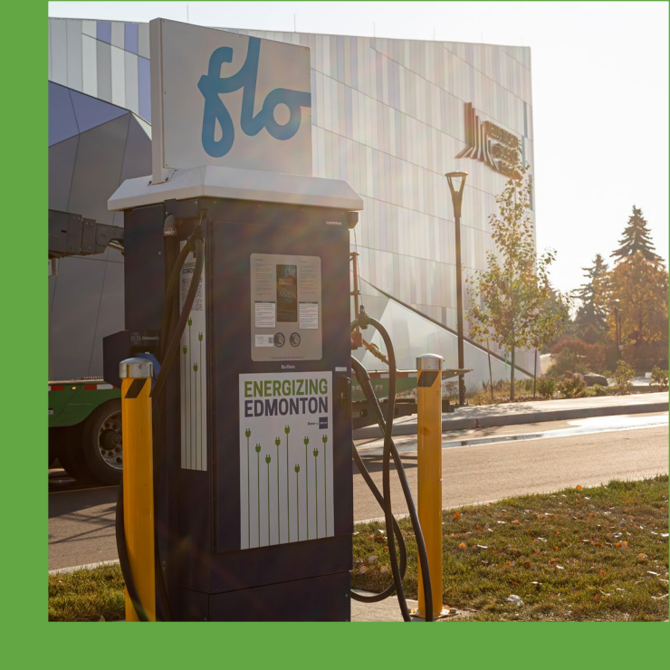
Encor by EPCOR installed 24 electric vehicle chargers — free to users in Edmonton, AB.
