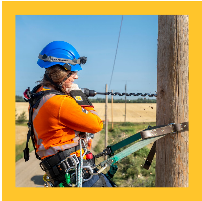
A power line worker prepares for the installation of electrical equipment in Edmonton, AB.
