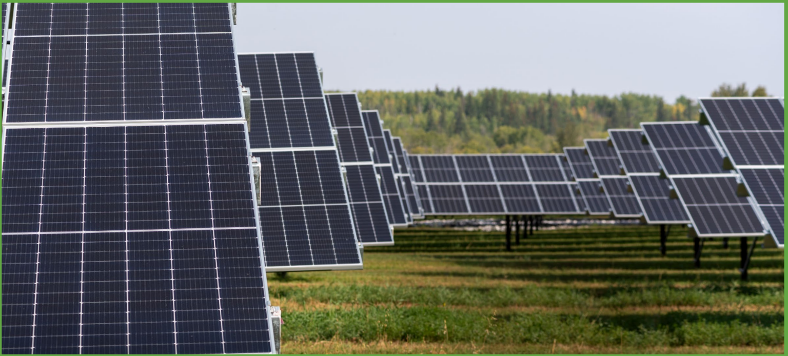
The k̓isik̓aw p̓isim solar farm now powers plant operations at the E.L. Smith Water Treatment Facility in Edmonton, AB.
